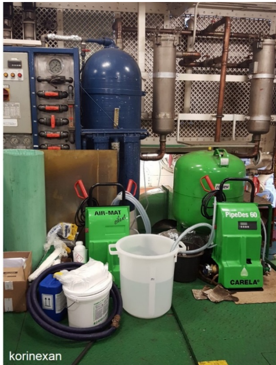
Equipment for cleaning on board
